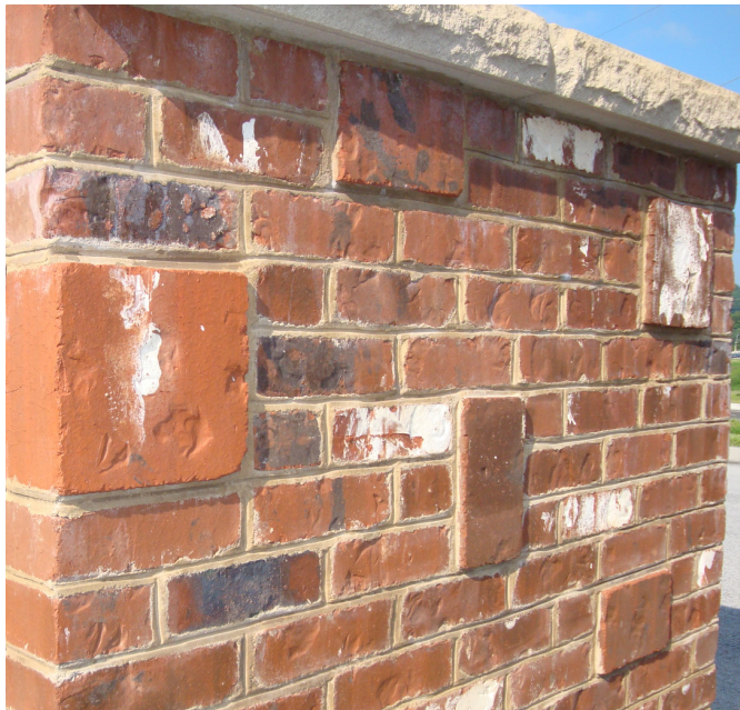
Figure 1 Here the Double and Triple units have been projected 1/2" out from the surrounding half and standard units. (Woodrose Park shown.)
