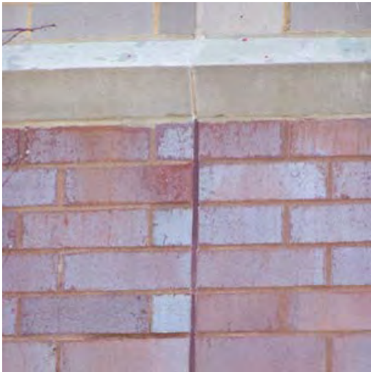
Figure 8: Change sealant color within the vertical joint to match changing unit colors up the height of the wall.
