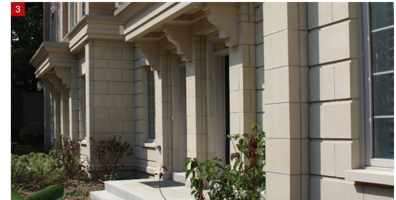
1. Custom Arch and Post units, Bullnose| 2. Bullnose and custom detail | 3. Chamfers and Sills
