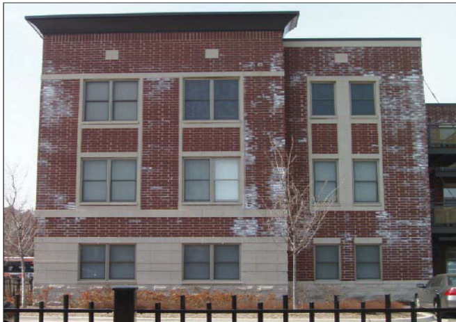
Photo 1: New Building Bloom. This type of efflorescence may begin before construction is completed.
