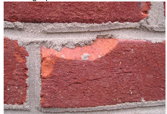
Figure 2: Mortar present on face of chipped brick
