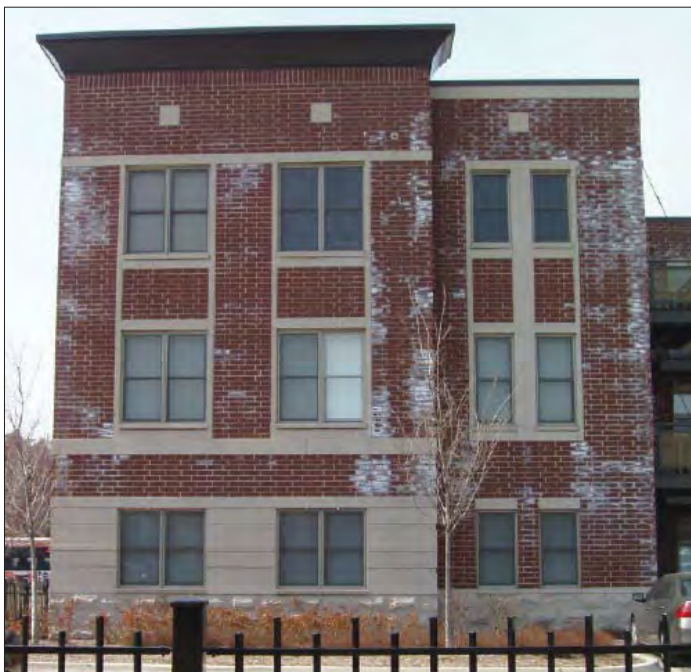
Photo 1: New Building Bloom. This type of efflorescence may begin before construction is completed.
