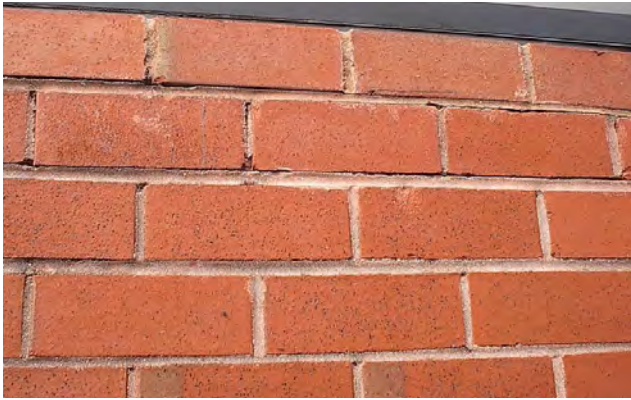
Photo 1 Mortar Joints in Need of Repointing
